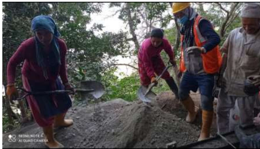
Ms. Gita Bhujel preparing concrete mix for the construction of Simle irrigation canal
